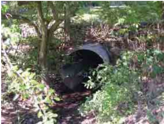
Zone 3 – undersized culvert
